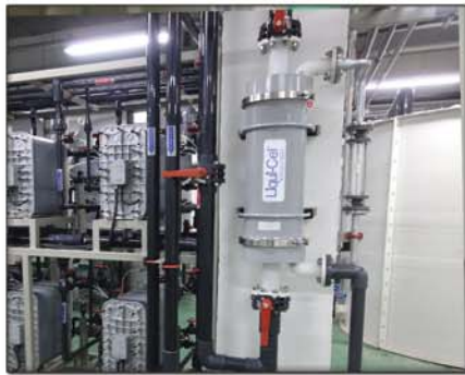
10-inch Oxygen Removal System
