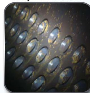
Pitting In Boiler Metal Surface
