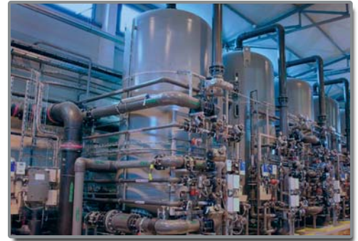
Mixed Bed Demineralizer for a Power Generation Facility
