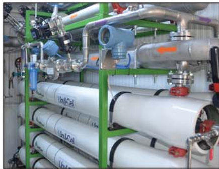
8-inch Mobile Deox System
