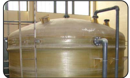
Chemical Storage Tank
